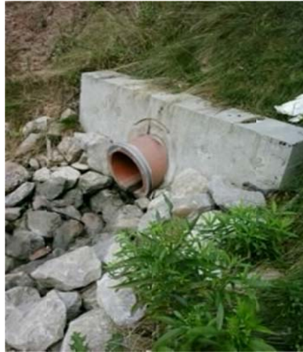
Figure 1. Example indication of a stormwater conveyance with an outfall location.
